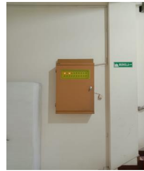
Gambar 14. Panel Lampu Penerangan Laboratorium EBT
