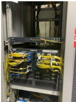
Gambar 4. Optical line terminal
