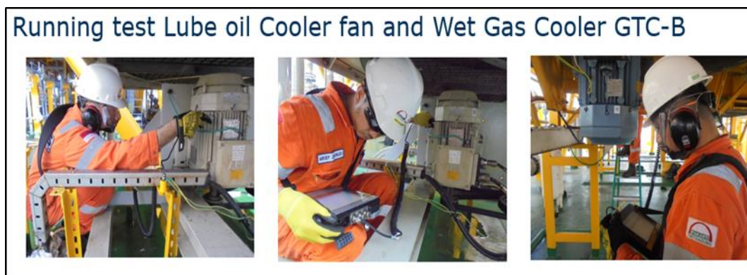
Gambar 2.1 Check Vibrasi Lube Oil Cooler fan dan Wet Gas Cooler GTC-B
